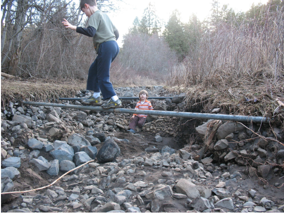
Our driveway 3/7/14 (Before the flood, these pipes were buried under the driveway)
